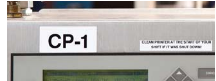
Control Panel & Electrical Panel Labels
